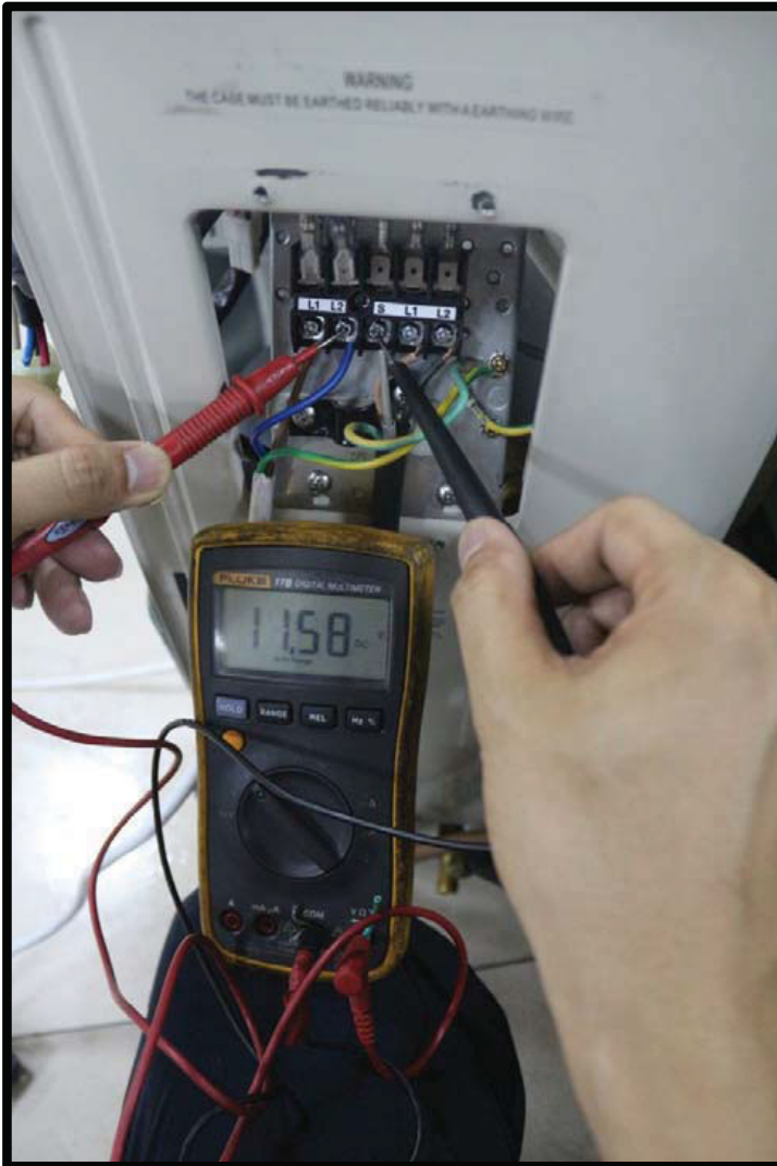
Fig. 27 – Test the DC voltage
